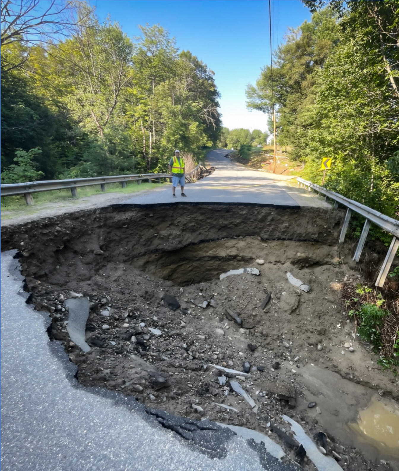
Flood damage on Woodman Hill Road in Jay, Maine, after heavy rainfall in summer 2023. Photo credit: Murray Carpenter, Maine Public Broadcasting Network. ( https://www.mainepublic.org/climate/2023-08-07/maine-has-been-hit-by-an-unusually-high-number-of-flash-floods-this-summer-straining-small-towns )
